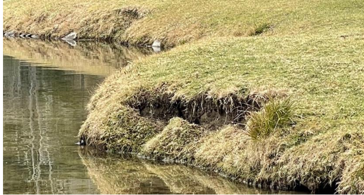
Shoreline Failure: Lawn down to the lake with bank slumping
